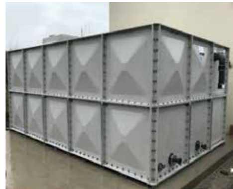
Grey Sprinkler Tank Example Image
